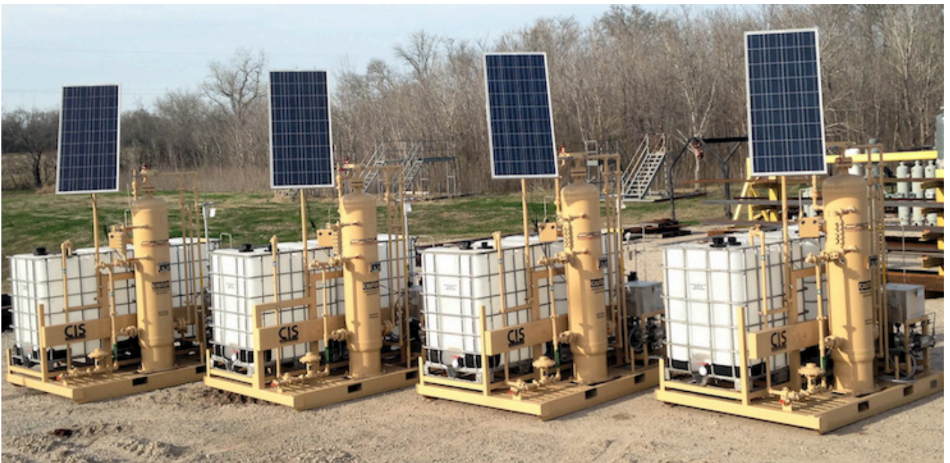
A totally redundant PLC-operated injection system can be controlled remotely or locally
